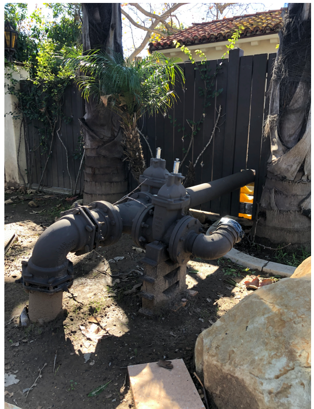
Photo 8: Looking South along Channel Drive showing above grade temporary piping.
