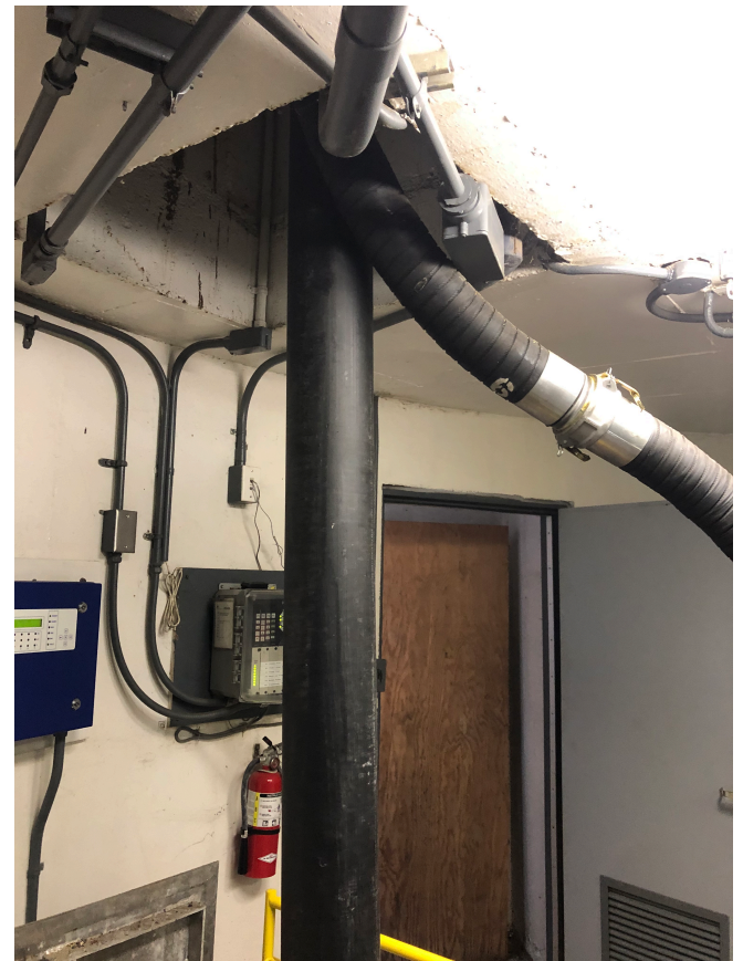
Photo 4: Mid level showing temporary piping through dry well shaft.
