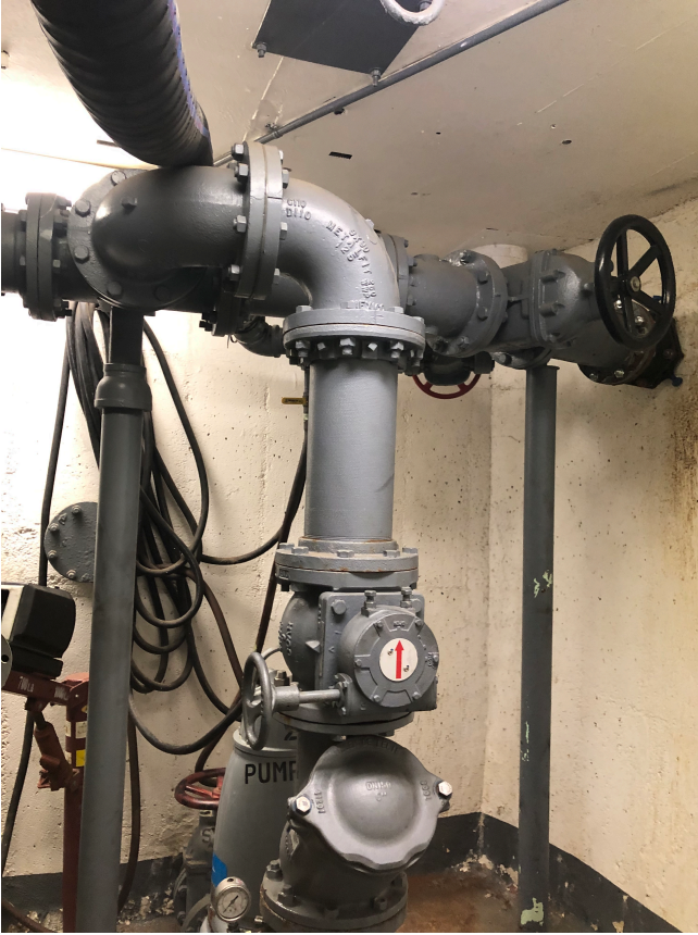
Photo 1: Lower level showing original discharge location through the wall and out of dry well.
